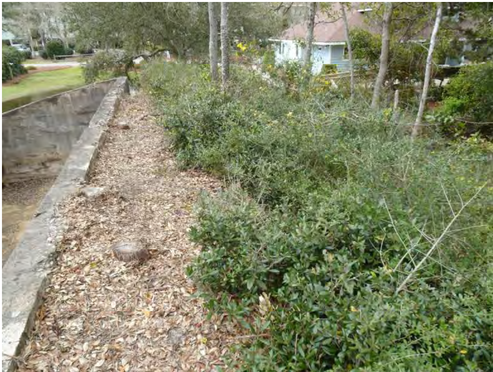
Photo B. Current condition with vegetation encroaching the rifle target pit.
