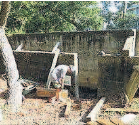
Okey Tucker makes a retaining wall before placing the concrete steps down into the pit.
