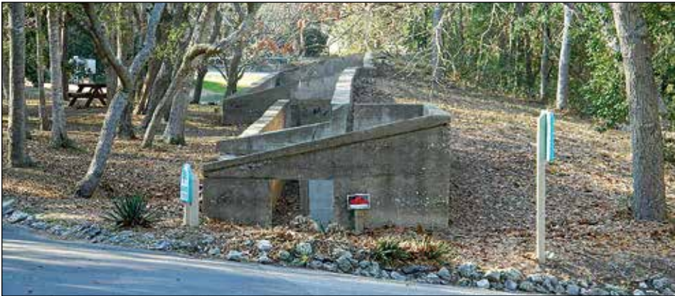
The 184-foot-long Fort Caswell Rifle Range wall is shown from the east side where the center wall is tilted inward displaying the need to stabilize it before it collapses.
