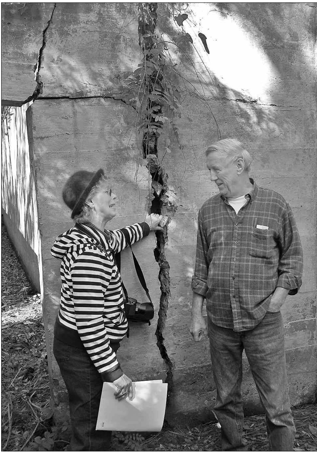
Photos by Lee Hinnant Ron and Norma Eckard examine the crumbling lintels inside the rifle range. Stabilizing the decay is the first priority.
